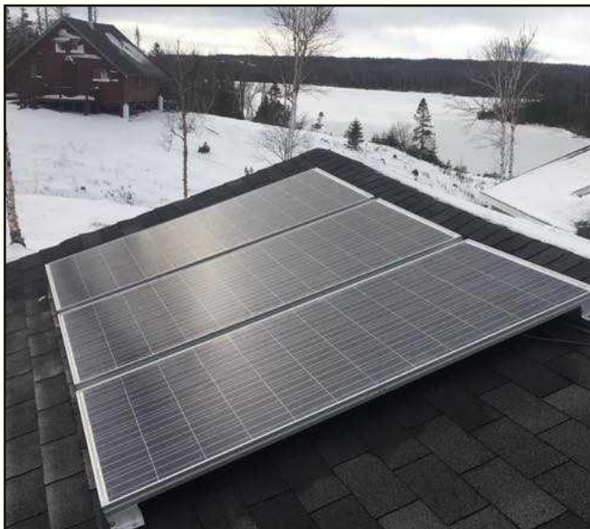
A roof-mounted solar panel system
